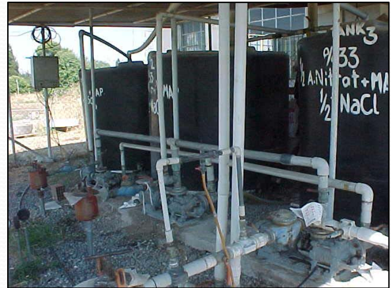
Fertilizer and Irrigation Tanks
